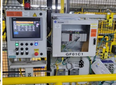
Global Standard Control Panel
