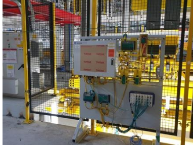
Global Standard Control Panel
